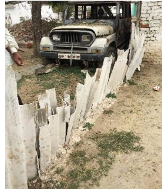
Asbestos sheet and waste being used as part of house construction
